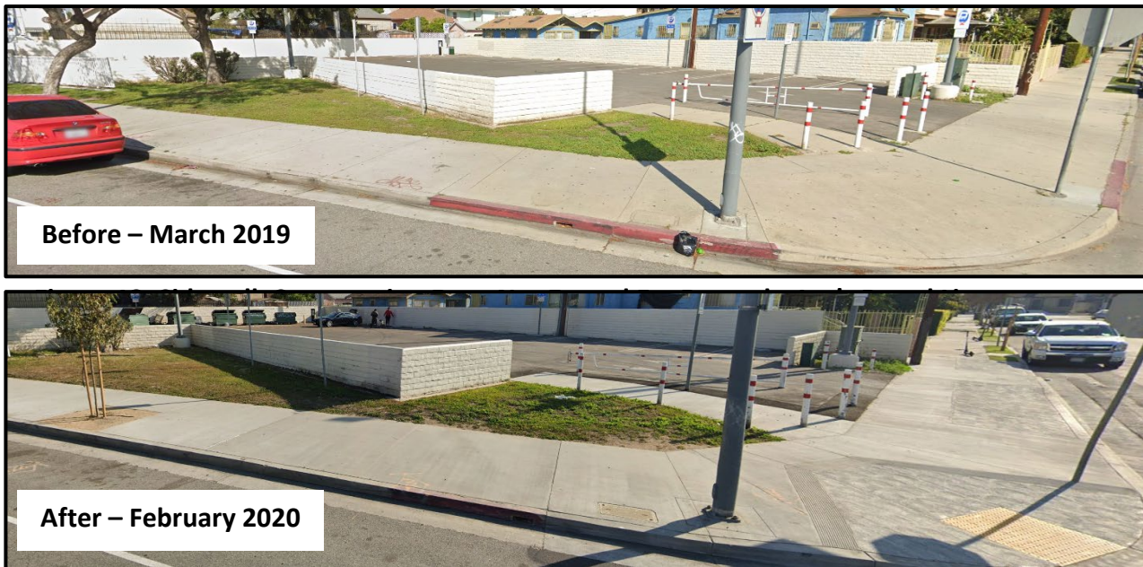
Figure 11. Repairs Include Every Aspect of Non-Compliance with Accessibility Standards
