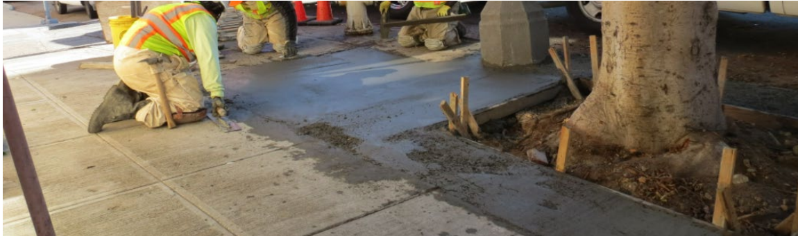
Figure 10. San Francisco's Sidewalk Programs Only Repair a Portion of the Sidewalk
