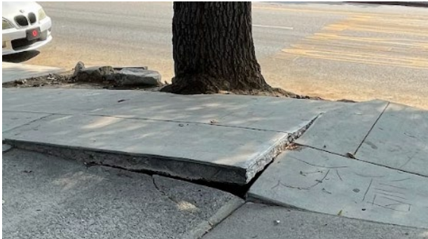
Figure 21. Previously Repaired Sidewalks Can Come into Conflict with Trees Again
