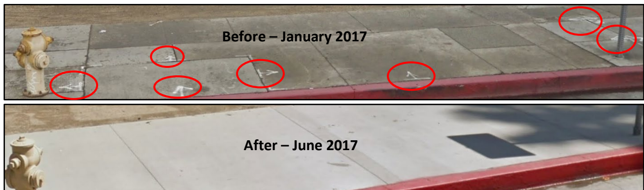
Figure 8. Non-Compliant Sidewalks are Marked for Removal and Replacement
