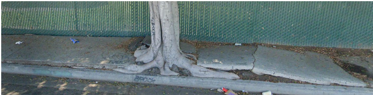
Figure 1. Broken Sidewalks Throughout Los Angeles Impede Pedestrian Traffic
